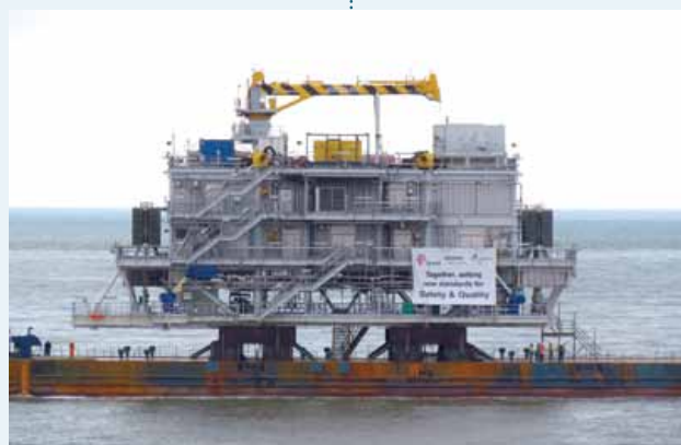
Dudgeon Offshore Wind Farm Substation Platform
