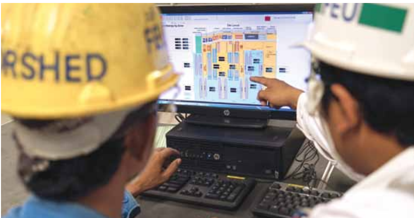
Power usage in the Tuas Boulevard Yard is monitored and managed with a Land-based Energy Management System
