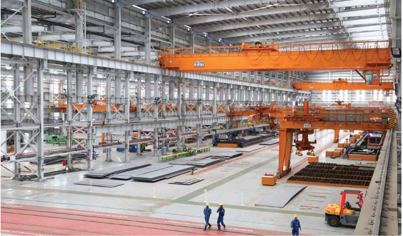
Sky lights and ceiling louvres in workshops significantly reduce the need for lighting and mechanical ventilation
