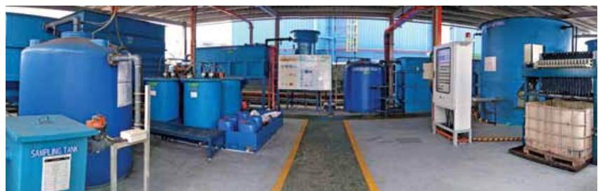
Waste water treatment plant at the Sembcorp Marine Tuas Boulevard Yard
