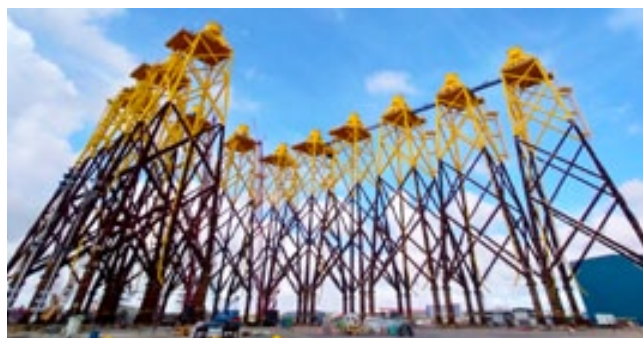
Fabrication of 15 wind turbine jacket foundations for the Formosa 2 Offshore Wind Farm in the Taiwan Straits
