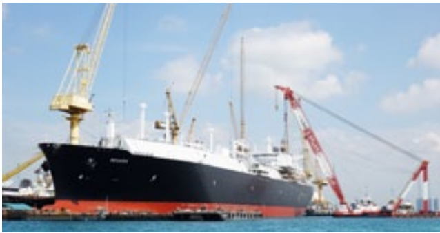
Performing LNG reliquefaction plant retrofits to enhance vessel fuel efficiency for greener operations
