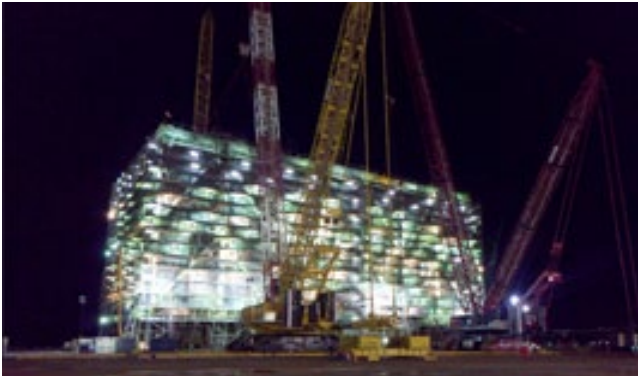
Work is in progress for the Sofia Offshore Wind Farm Offshore Converter Platform
