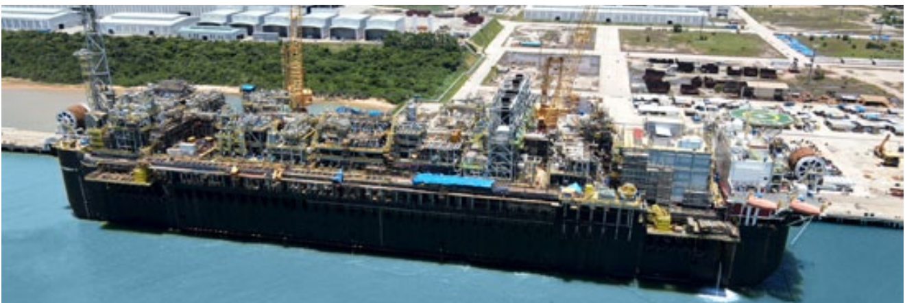
Completion of modules fabrication and integration for newbuild FPSO P-71 at our EJA Yard in Brazil
