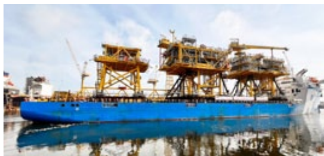
Delivery of two wellhead topsides, a riser topside and two bridges for the Tyra West facilities marks the completion of the Tyra Redevelopment Project following completion of the Tyra East production topsides and bridges in 2021
