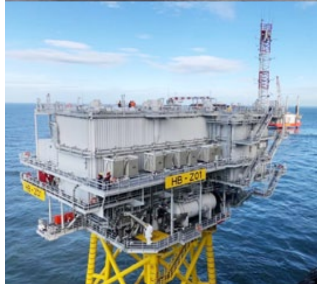
Completion of Hornsea 2 Offshore Wind Farm Offshore Substation and Reactive Compensation Station fabrication, offshore hook-up and commissioning in the UK North Sea.
