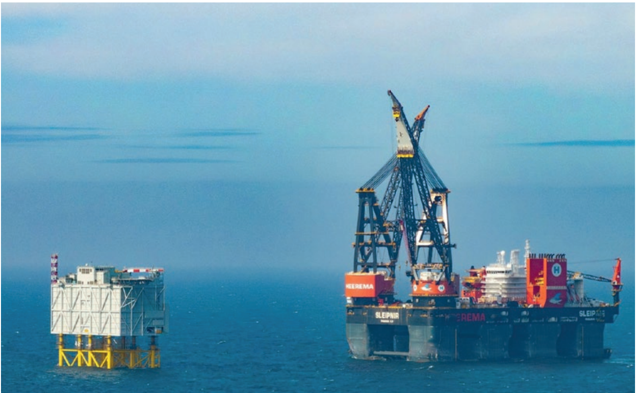
Successfully installed 13,000-tonne topside for RWE Renewables' 1.4GW Offshore Converter Platform (left in picture) – the heaviest lift in the offshore wind industry – at the Sofia Offshore Wind Farm
