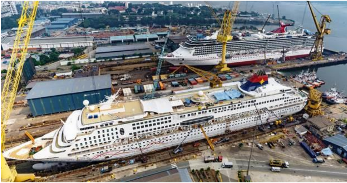
Concurrent repair of Superstar Gemini for Star Cruises and Carnival Spirit for Carnival Cruise Line at Sembcorp Marine Admiralty Yard in August 2015
