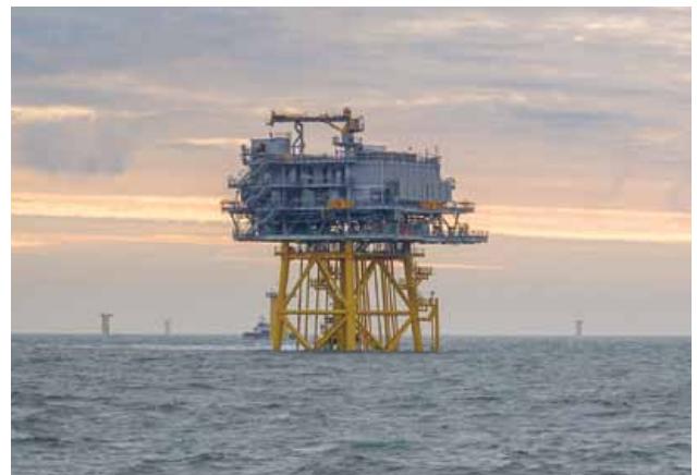
Offshore substation platform deployed for the Dudgeon Offshore Wind Farm in the UK North Sea
