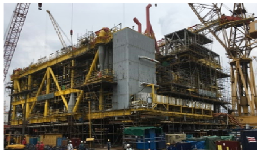
Wellhead Head Platform
