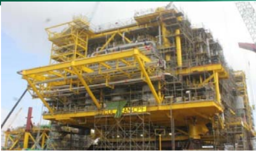
Central Processing Platform + GCM
