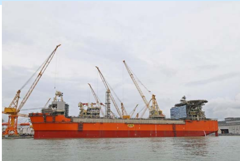
Project: Turnkey FSO newbuilding comprising engineering, procurement, construction and commissioning, including installation and integration of turret and topside modules Customer: MODEC Operation: Maersk Oil's Culzean field, UK North Sea
