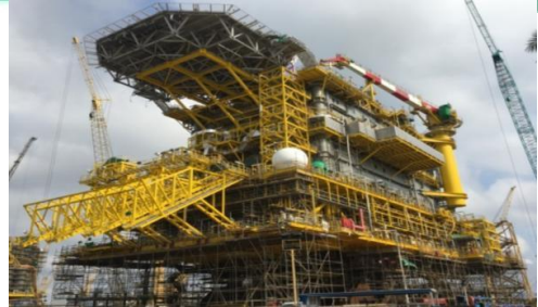
Utilities & Living Quarter topsides
