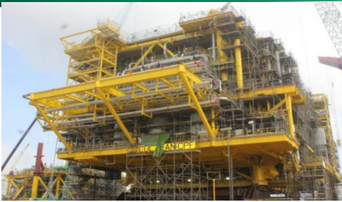
Central Processing Facility + GCM
