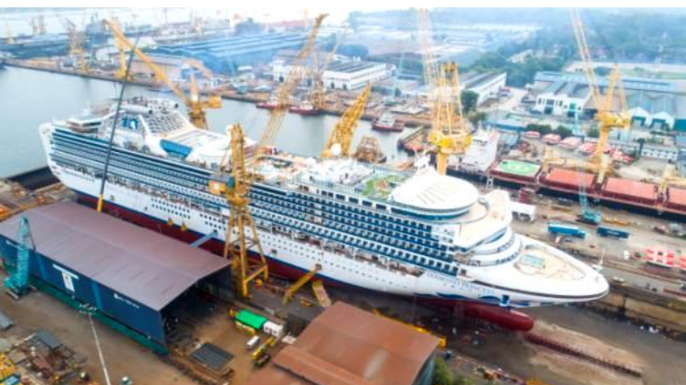
Repairs and installation of scrubbers on Diamond Princess for FCC partner Princess Cruises
