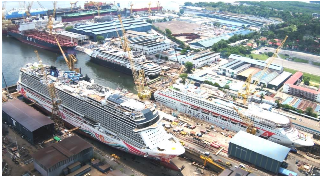
Extensive refurbishment of Norwegian Joy for Norwegian Cruise Line, major refit of Karnika for Jalesh Cruises as well as repairs of Vasco da Gama for Global Cruise Lines Ltd
