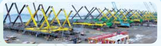
Fabrication of 15 wind turbine jacket foundations for the Formosa Phase 2 Offshore Wind Farm
