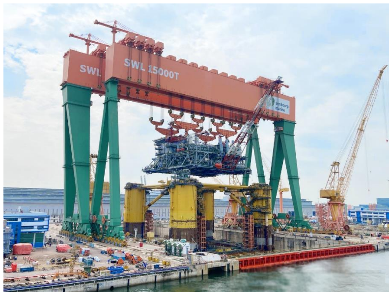
Integration of Vito topsides with the FPU hull ( Photo: SCM, all Rights reserved )
