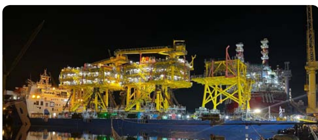
Delivered final phase of the Tyra Redevelopment Project with the completion of two wellhead topsides, one riser topside and two bridges for the Tyra West Field in 2022
