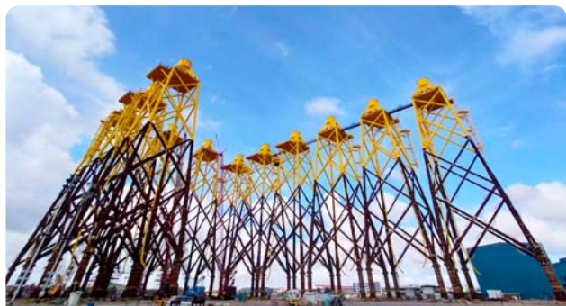
Fabrication of 15 wind turbine jacket foundations for the Formosa 2 Offshore Wind Farm
