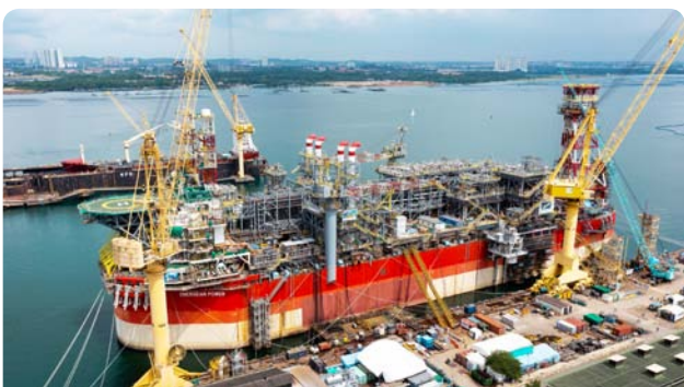
Energean Power newbuild FPSO for the Karish Field
