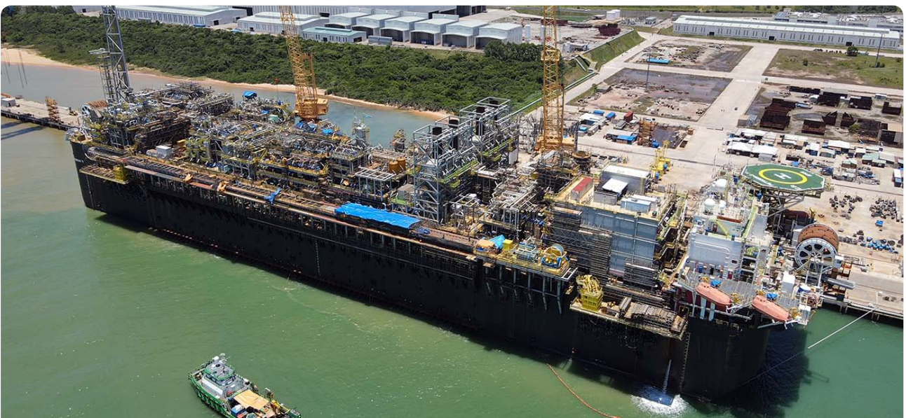
P-71 FPSO modification and topside modules work underway in our Brazil yard
