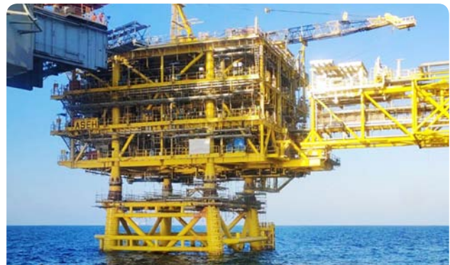
Offshore works in progress on two wellhead platforms and bridges for the Gallaf Batch 2 Project at the Al-Shaheen Field
