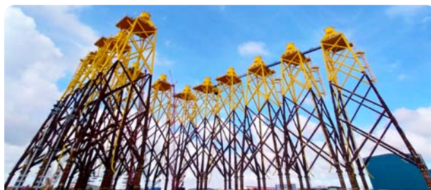
Completed fabrication of 11 wind turbine jacket foundations for the Formosa 2 Offshore Wind Farm in 2022, following the sailaway of four units in 2021
