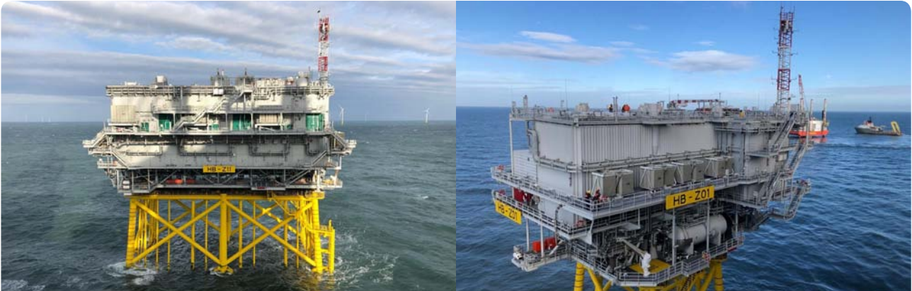
Offshore hook-up and commissioning of the Offshore Substation (left) and Reactive Compensation Station underway at the Hornsea 2 Offshore Wind Farm in the UK North Sea. The AC offshore substation is the largest of its kind ever built.
