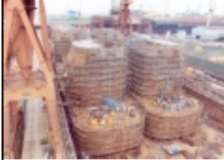
(1) Lower hull, consisting of 2 parts of pontoons & columns, constructed separately in another Drydock
