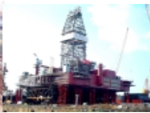
(2) The Upper Hull, measuring 8.5m x 75m was built over a skid truss on land in front of the Drydock
