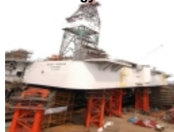
The 1 st unit Upper Hull built on skid truss in front of Drydock ready for the "Load-out and Mating-in-Dock" operations
